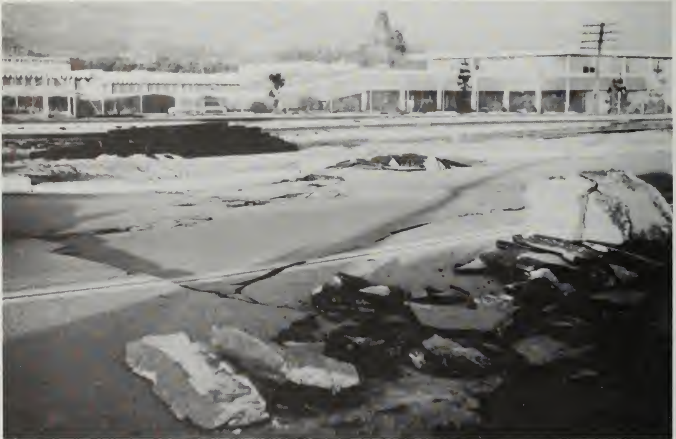
Liquefaction during the 1971 San Fernando earthquake caused serious damage to a Los Angeles County Juvenile Hall Facility. Prior knowledge of hazard potential can permit mitigation by site remediation or foundation design. Photo by Charles Real.
